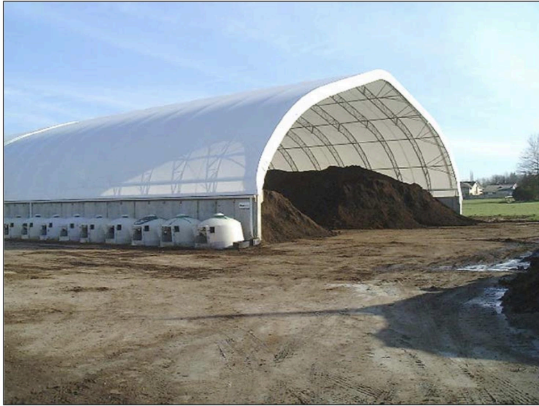
Figure 1: Hoop frame storage for solid agricultural waste, A covered structure used for manure, urine, bedding, and other biological wastes, typically cleaned out from animal pens and stalls (BC Ministry of Agriculture, 2015).
